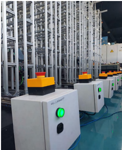
Figure 6. Local box for AGV in station
